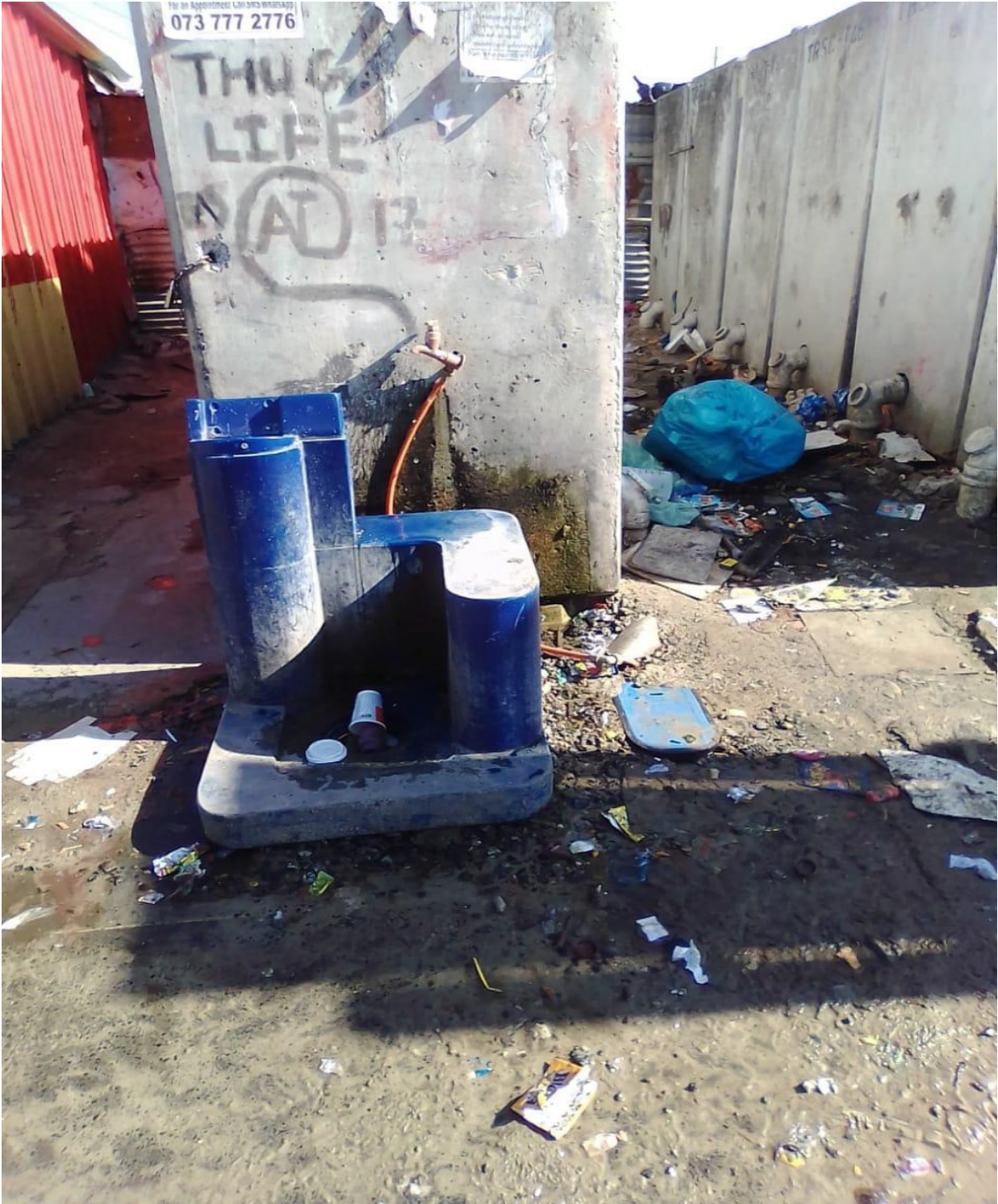
Figure 16: Communal taps and toilets that have not worked for months (Photo taken by Minga, 21 July 2020).
