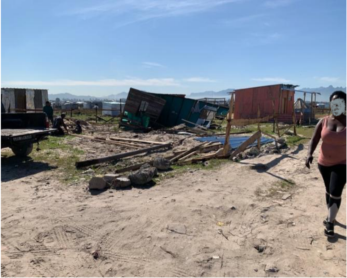
Figure 25: Residents are busy rebuilding their shacks after demolition by the law enforcement (Photo taken by Minga, 29 September 2020).
