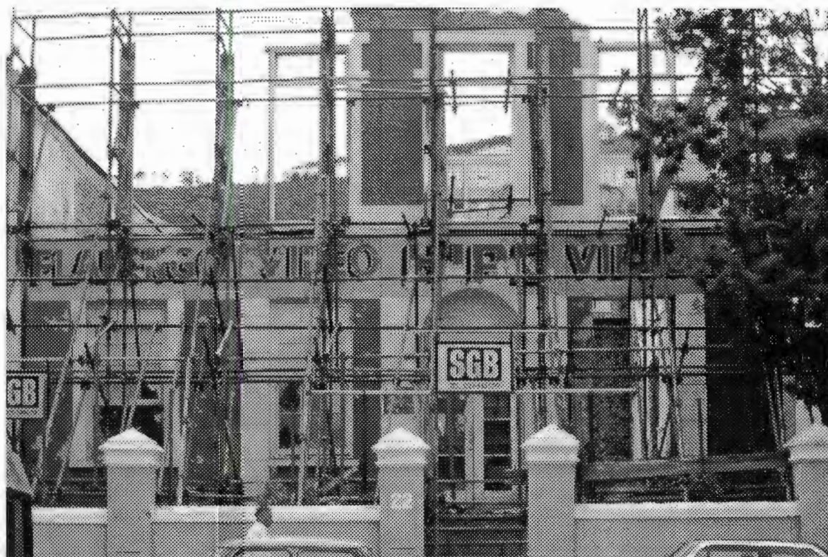
22 Kloof Street: the final stages of collapse (photographed October 1989)
