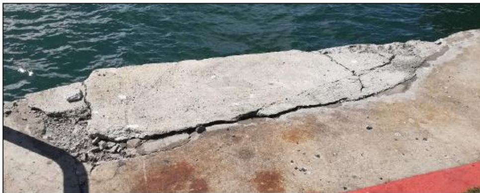
Figure 49: A piece of loose concrete along the cope edge
