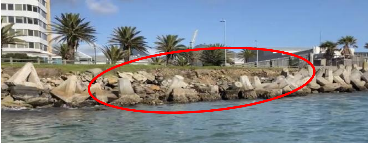
Figure 4.7: Excessive erosion on a seawall section at the Port of Cape Town (Picture supplied by TNPA)
