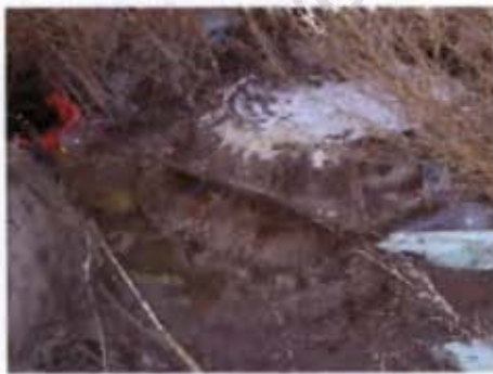
W: Waterworks, leaking sewerage manhole
