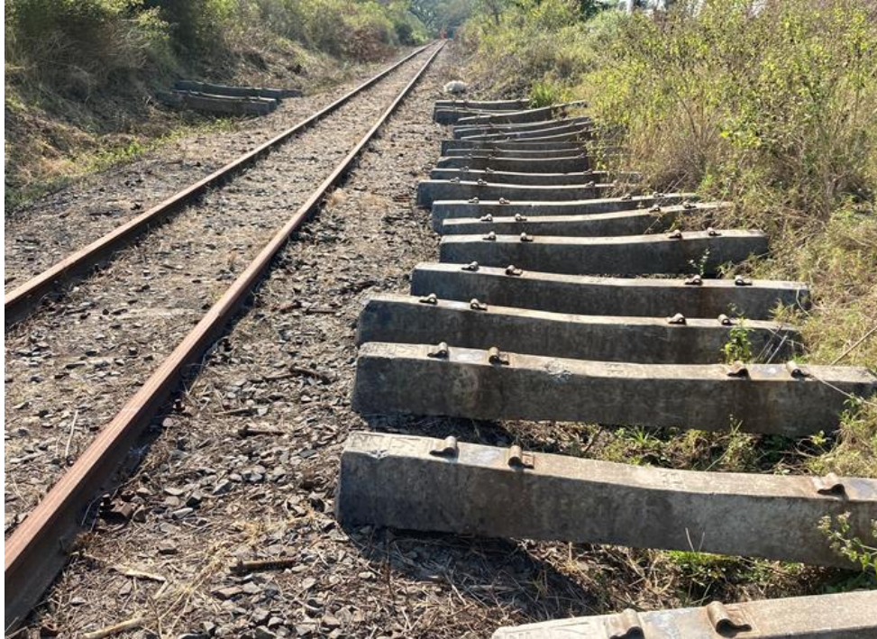
Figure 1.3: Concrete sleepers placed alongside the wooden sleeper track in preparation for replacement
