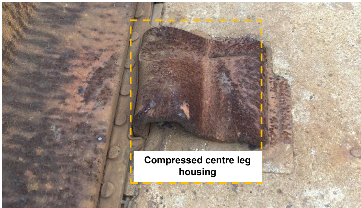
Figure 5.3: Deformed cast iron shoulder due to impact from a derailed locomotive wheel
