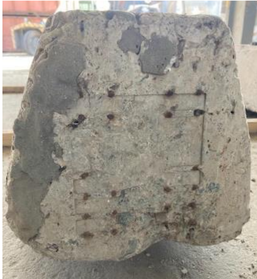
Figure 4.3: Substandard patch repair observed on the southern side of sleeper number 6
