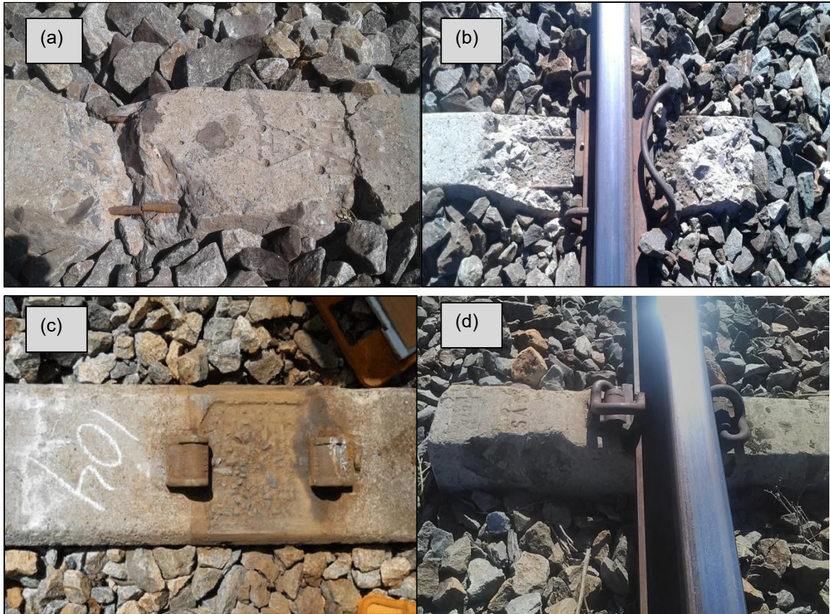
Figure 3.2: (a) A sleeper exhibiting significant cracking and compromised steel wire due to stress corrosion (b) Rupture around the rail seat position (c) Rail seat abrasion (d) Chipped concrete sleeper on the shoulder (Lutch, Harris and Ahlborn, 2009)
