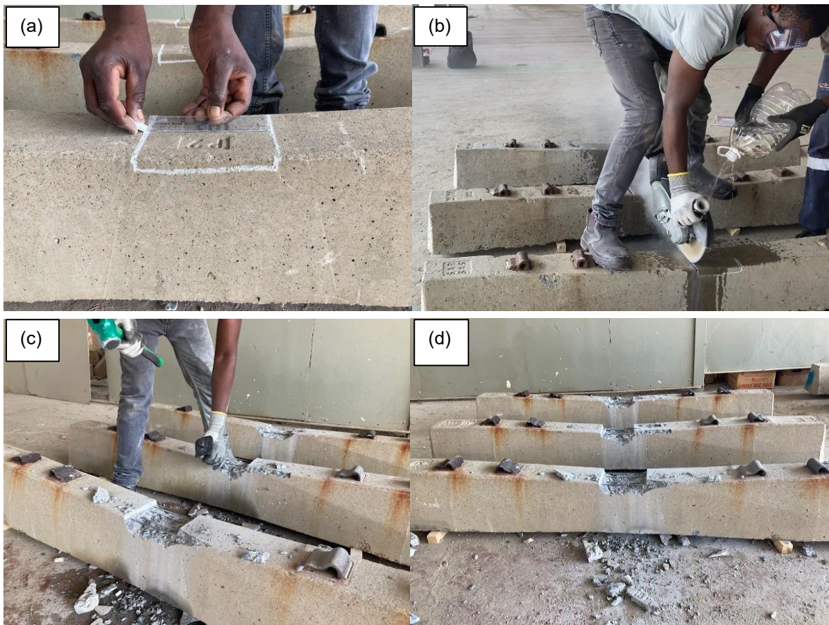
Figure 3.5: (a) Marking of the portion of the concrete removed with a 150 mm ruler (b) Grinding of concrete at the marked transverse contours (c) Concrete removal using a 2.7 kg hammer and bull-pointed chisel (d) Exposed prestressed wires.
