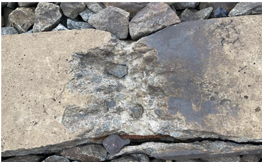
Figure 5.1: Significant concrete chipping and spalling have occurred, resulting in the exposure of corroded prestressed wires.
