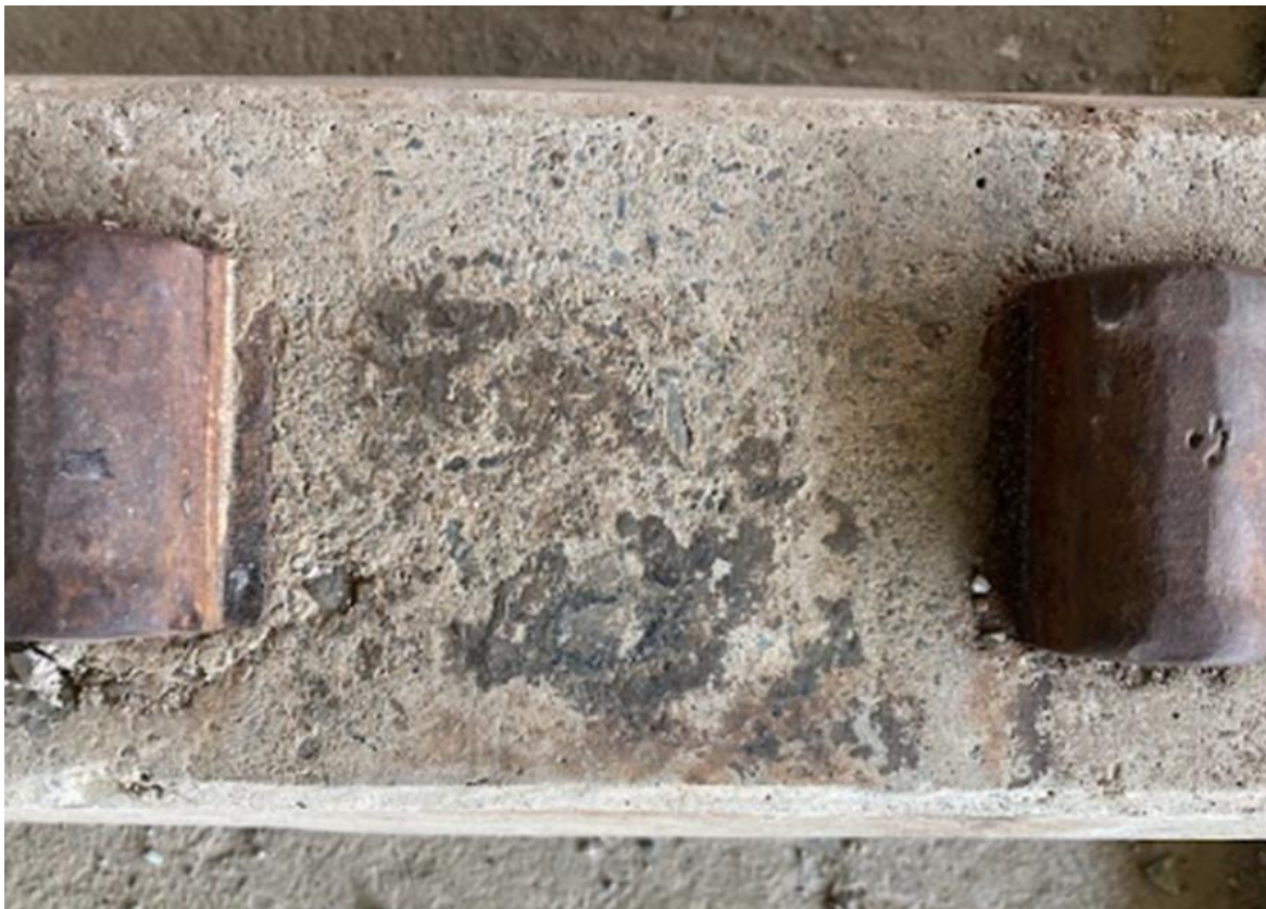
Figure 4.2: A typical slightly abraded rail seat area exhibiting residual rail-sleeper pad material
