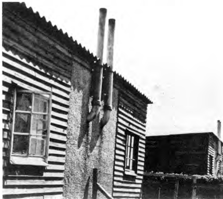
Illustration 3.9 Kwaford house built from packing cases donated by the Ford Motor Company (SA Panorama).
