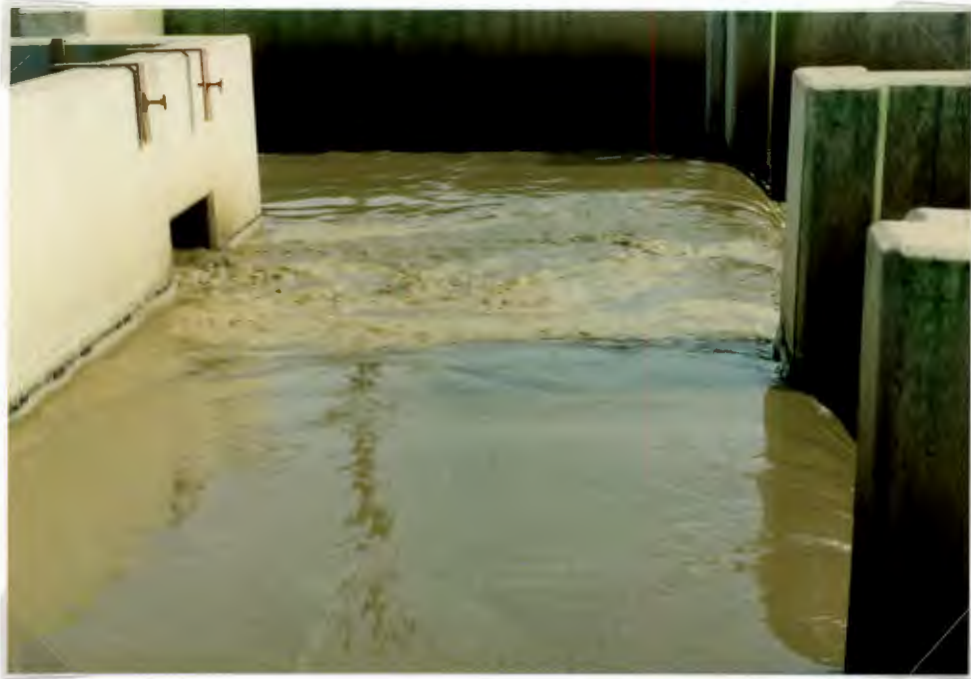
Photo 7.3: Preferential flow and Nocardia foam/scum travelling toward one weir of the mixed liquor splitter box (refer to Photo 7.2).
