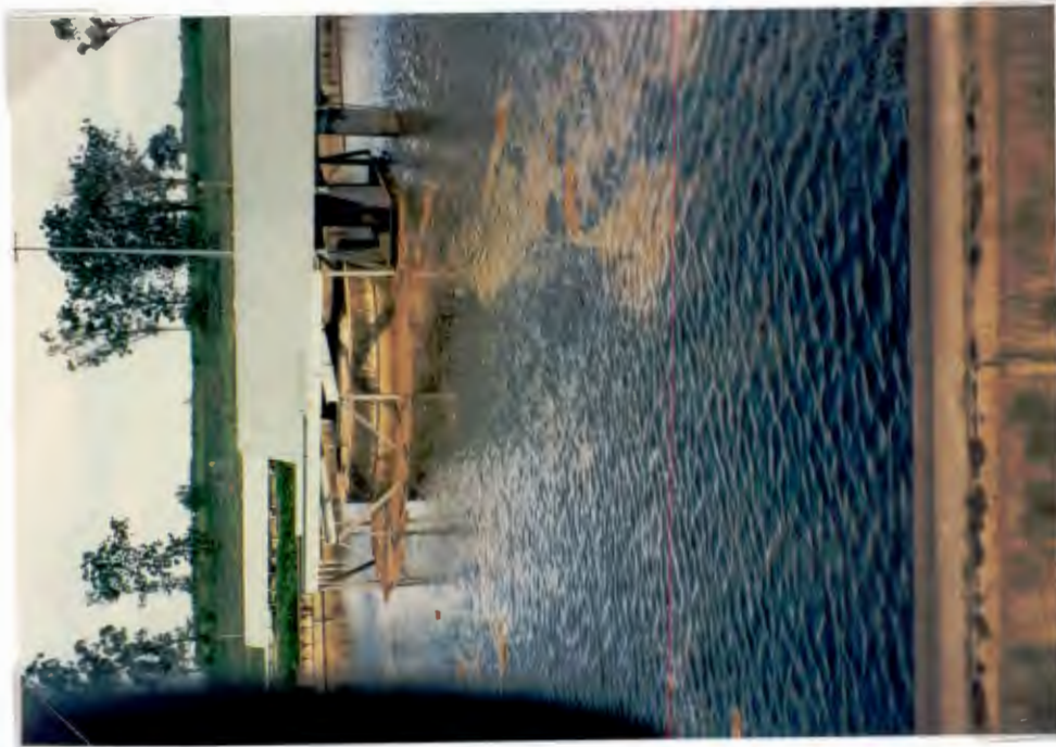
Photo 7.6: Detail of scum carry-over from SST A in the direction of prevailing wind making it difficult to obtain a representative sample of effluent suspended solids (see also Photo 6.9).
