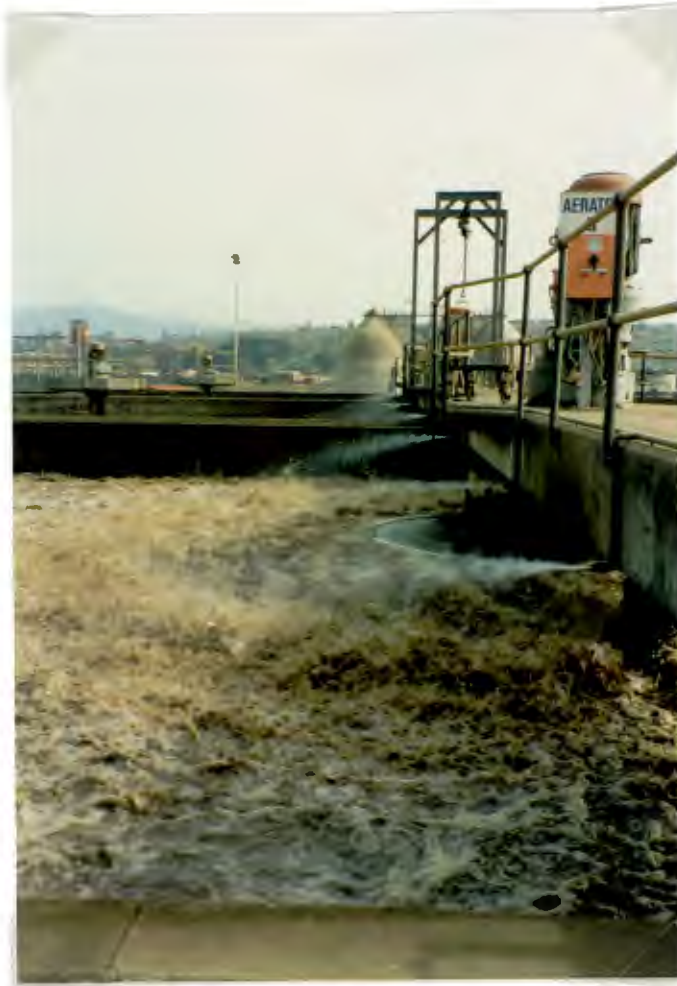
Photo 6.5 : Use of aeration basin high pressure water sprays in an attempt to break up foam and scum on aeration basins.
