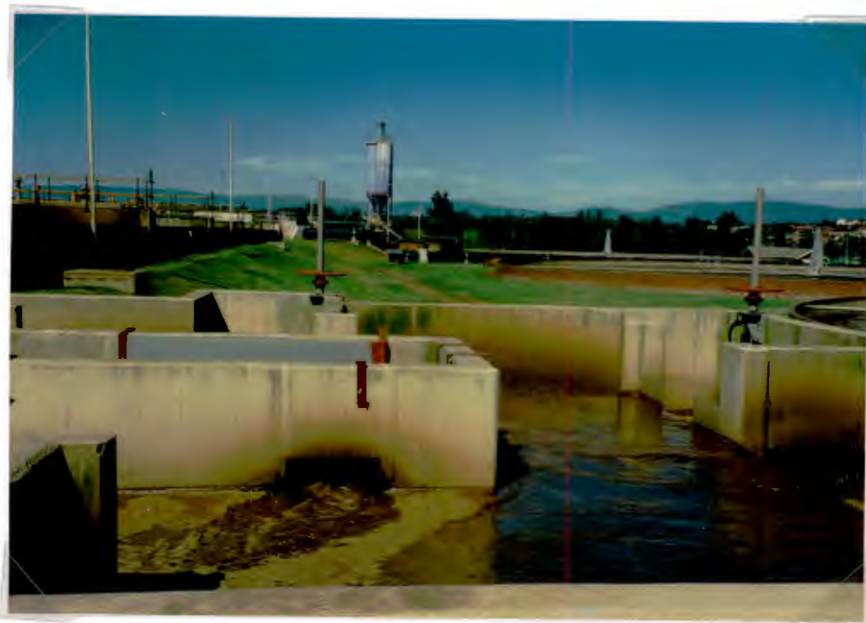
Photo 7.2: Mixed liquor splitter box showing one of three 500mm square of scum holes, considered to be too large due to tendency to bias flow in the direction of the nearest weir splitting flow to one secondary clarifier. Temporary baffles are shown, used to reduce flow via scum holes and equalise split to clarifiers. This practice tended to trap Nocardia upstream.
