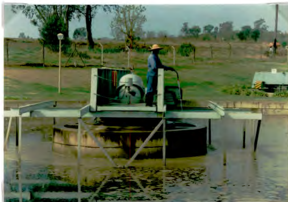
Photo 6.8: The central skirt baffle retrofitted to old SSTs (A, D and E) served to improve clarifier performance by expanding the central flocculation well. Despite being approx. 10 mm below top water level, the baffle set up flow conditions which trapped Nocardia scum. Hosing with water helped to dislodge the scum but this aggravated the solids carryover problem.
