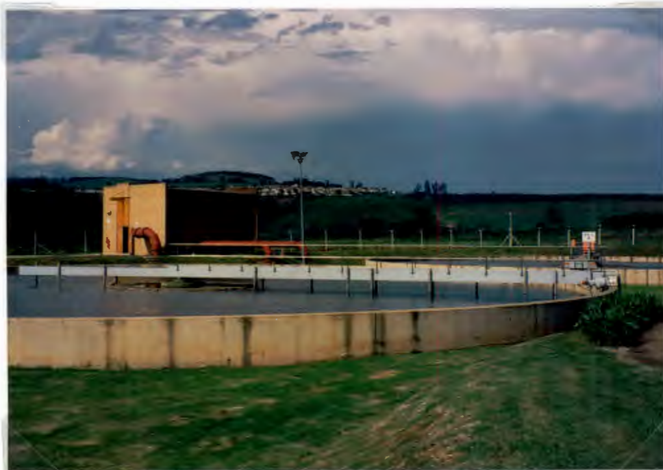
Photo 6.12: "New" secondary clarifier (SST B) virtually free of scum on 14/1/97. The return activated sludge pumphouse is situated in the background.
