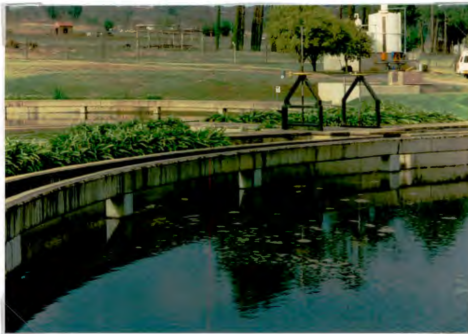
Photo 6.7: Scum carryover. Solids floating out over the surface of one of the secondary settling tanks (SST A) and contributing to the secondary effluent solids and pathogen load.
