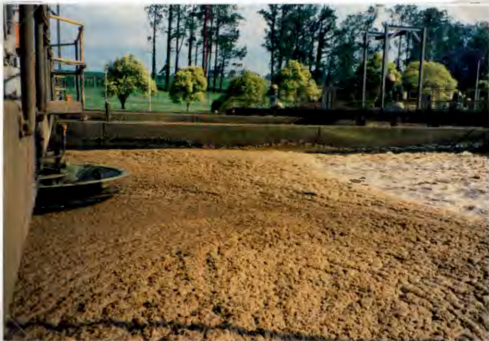
Photo 6.4: Foam covering an aeration basin with an aerator switched off.
