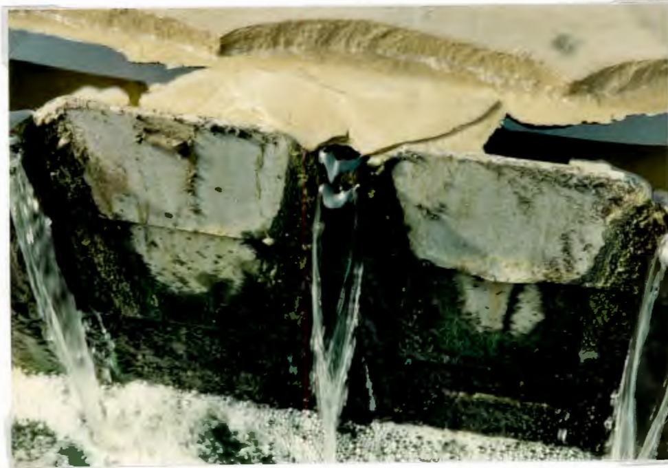
Photo 6.10: Detail of scum carryover problem at secondary clarifier overflow weir. The effluent itself is very clear but lumps of scum break off and pass over into the effluent launder.
