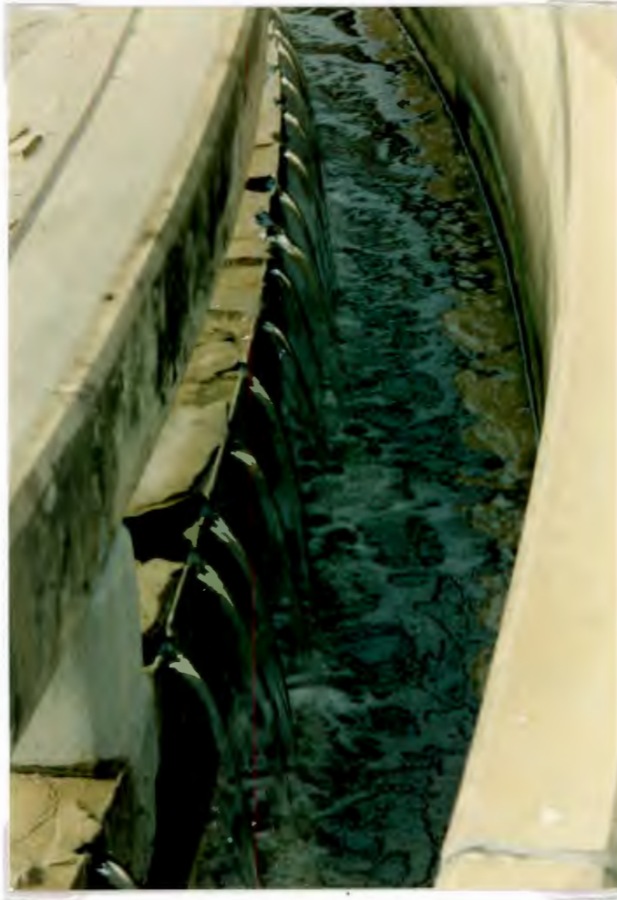
Photo 6.9: Oily scum carryover from secondary clarifier into effluent launder. Nocardia problem compounded by high influent concentrations of vegetable oil emulsions (trade waste).
