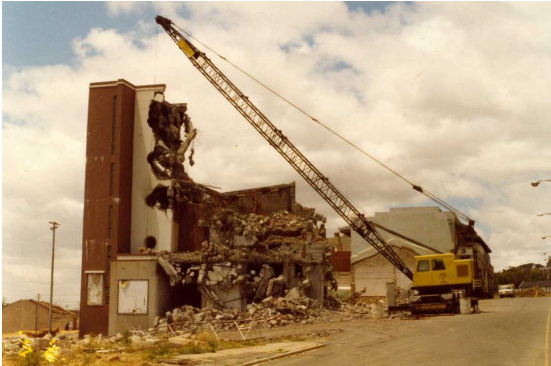
Figure 21: The demolition of Avalon Cinema in District Six (District Six Facebook page, Alex Lawrence, n.d)
