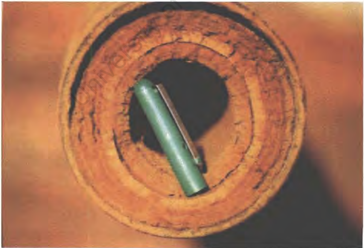
Figure 1 A clogged riser pipe showing the layering of precipitate inside the pipe
