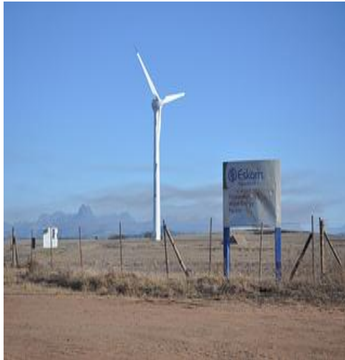
Figure 2.1: Klipheuwel experimental wind farm project
