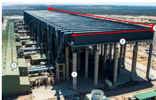
Figure 2-3: ACC at Medupi power station, South Africa (Augustyn, 2017)
