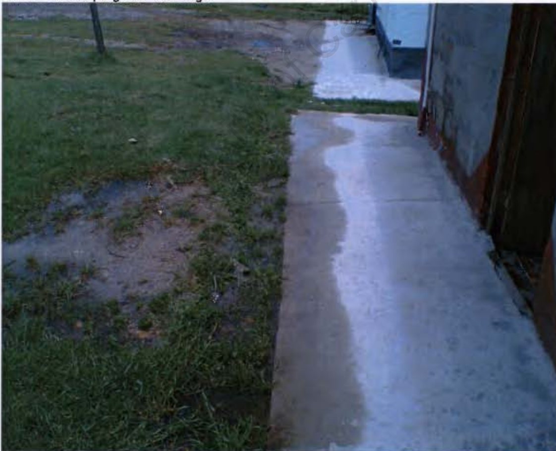
Figure 8.6 Example of the effectiveness of the concrete dipping floor in preventing ponding water from seeping into dwellings
