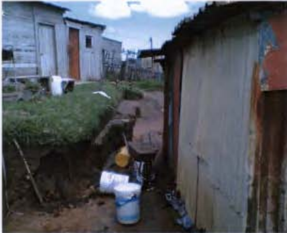
Figure 8.10 An Informal Dwelling that has Excavated a chunk of earth around the dwelling In an attempt to prevent seepage and ponding
