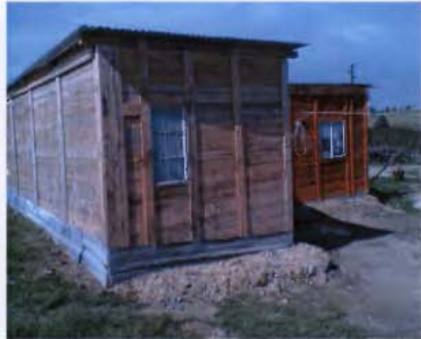
Figure 8.11 An Informal Dwelling that has Inserted corrugated iron sheets to the bottom of the dwelling & securing it with sand in order to prevent seepage
