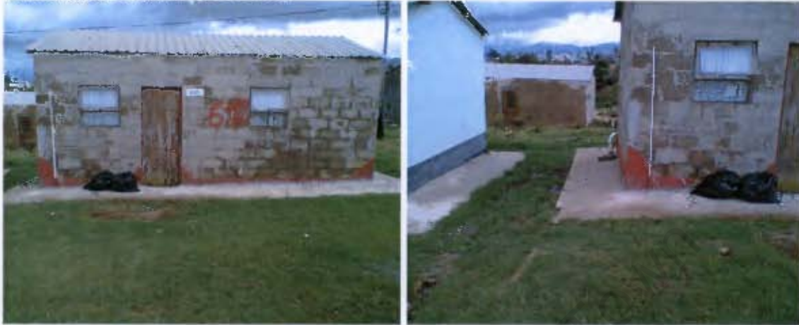
Figure 8.5 a (left) and b (right) Examples of dwellings with newly installed concrete dipping floor following the August 2006 events
