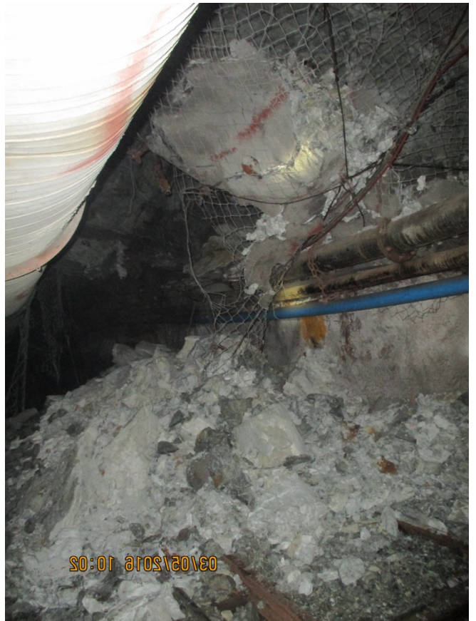
Photo 12: Typical tunnel underground after fall of ground
