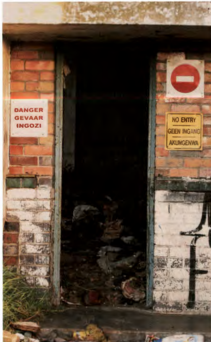
An entrance to the derelict building
