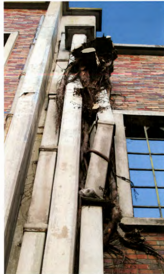
the roots of one of the trees that grew up the power station; inside a rain water down pipe
