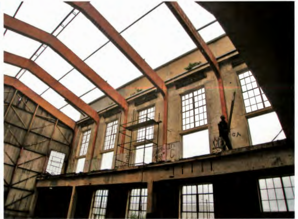
the massive, poetic, concrete rib-like beams used to support the roof structure
