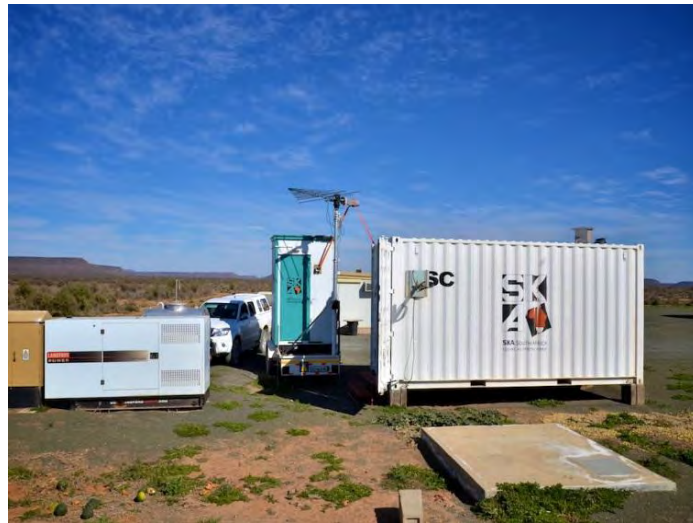
Figure 35 - RFI monitor antenna and ASC container at the KAT7 site
