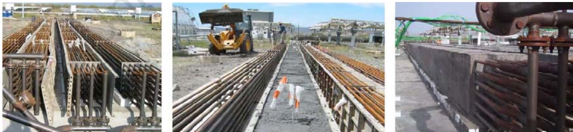
Figure 5.3.16: Pilot scale concrete storage system. Source: (DLR, 2008)
